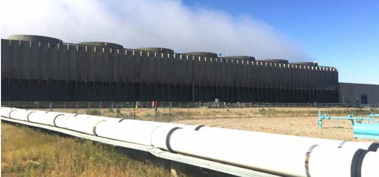
The evaporative cooling towers at the SaskPower Shand Power Station (Courtesy: SaskPower).
