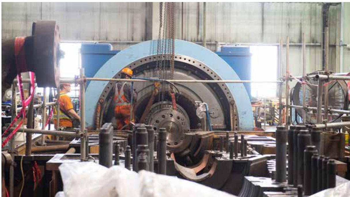
Inside the BD3 Power Generator during scheduled maintenance (Courtesy: International CCS Knowledge Centre).
