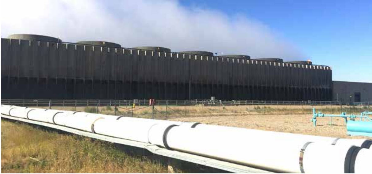
The evaporative cooling towers at the SaskPower Shand Power Station (Courtesy: SaskPower).
