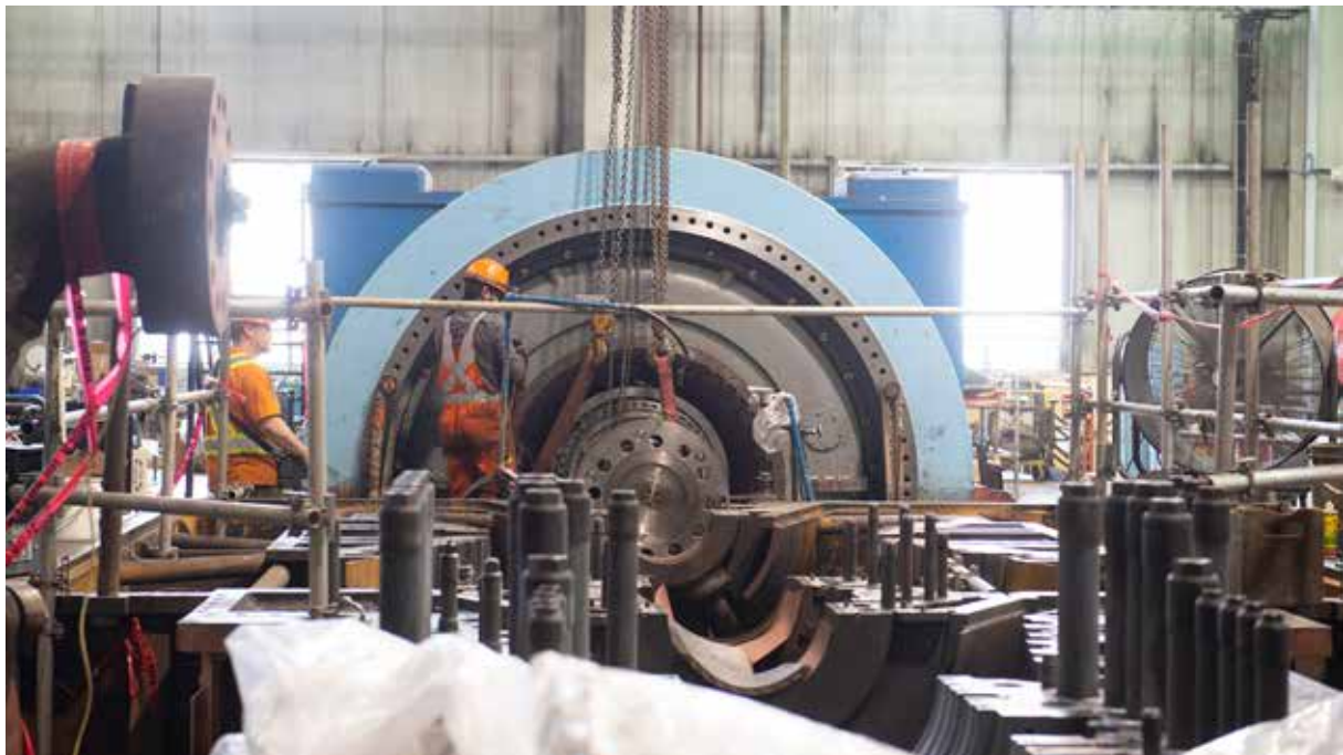
Inside the BD3 Power Generator during scheduled maintenance (Courtesy: International CCS Knowledge Centre).
