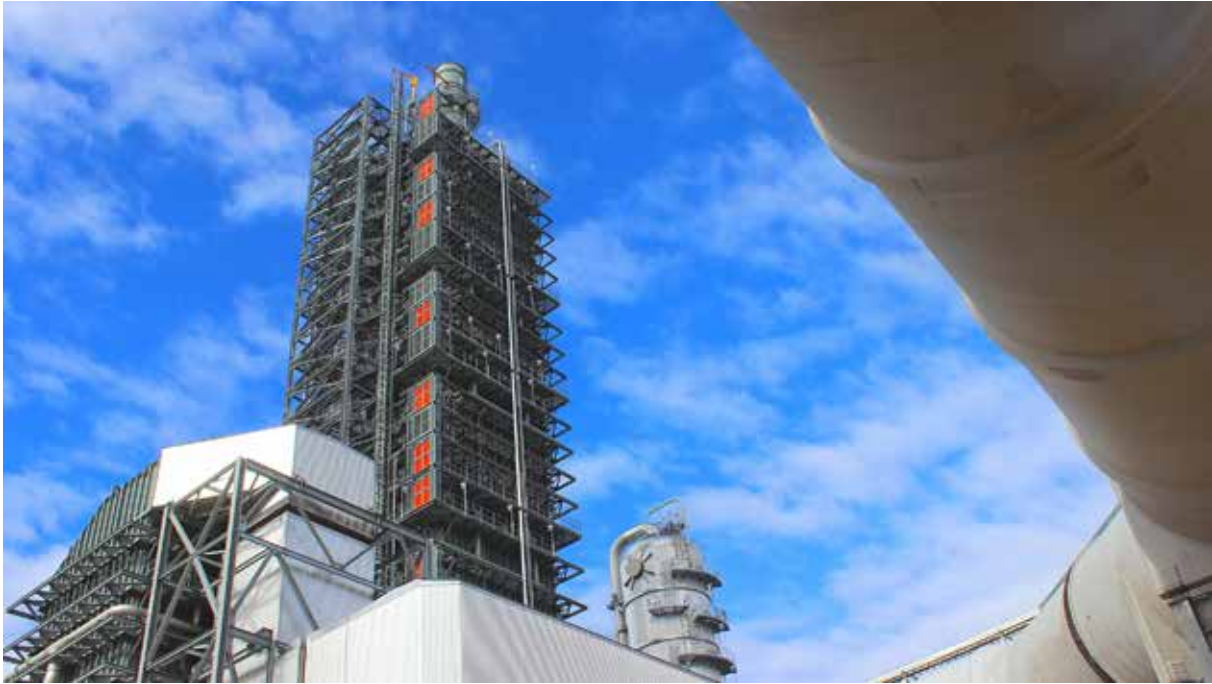
The Carbon Capture Facility at the Petra Nova WA Parish Power Station (Courtesy: NRG Energy).
