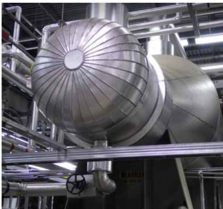
The kettle reboiler inside the Carbon Capture Test Facility at the SaskPower Shand Power Station (Courtesy: SaskPower)
